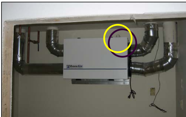
Photo 4 – Shows a sprinkler obstructed by a ceiling-mounted ventilator
