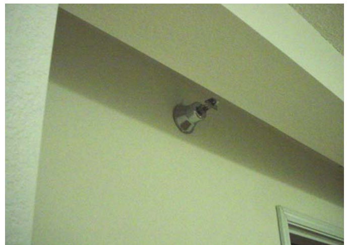
Photo 2 – A beam installed directly in front of this sprinkler obstructs its proper operation
