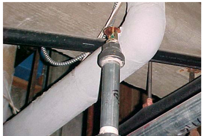
Photo 1 – Obstruction to proper sprinkler operation
