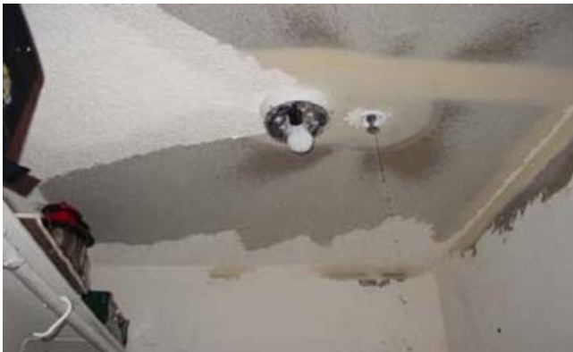
Photo 3 – Shows the obstruction pattern posed by a light fixture (note the “shadowed” area beyond the light).
